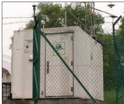
Photo 3: Continuous Air Quality Monitoring Station (DOE Photo Library)
