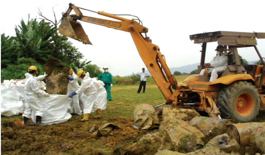
Clean up of scheduled waste at illegal dump site (DOE Photo Library)
