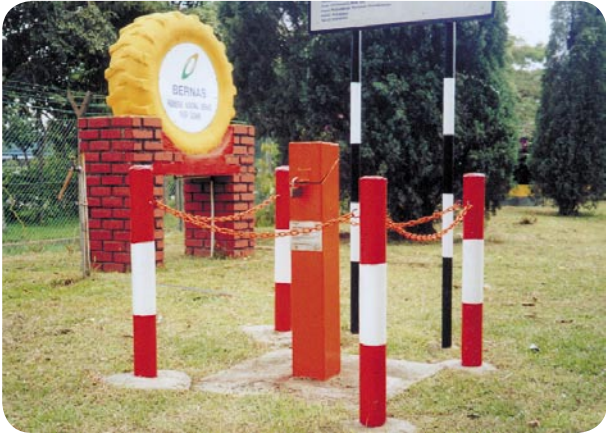
Gambarfoto 5.15 JAS: Stesen Pemantauan Kualiti Air Tanah Photo 5.15 DOE : Groundwater Quality Monitoring Station
