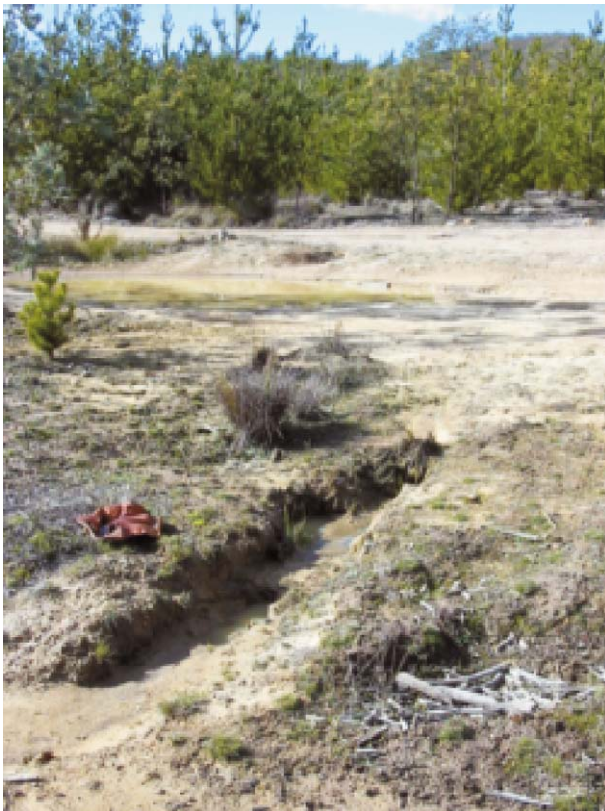
Figure 8 Erosion of the hillslope at road drainage outlets is a significant contributor to off-site sediment delivery in forested catchments. Large volumes of overland flow from road surfaces are discharged at single outlet points, often causing increased shear stress and the development of rills or gully erosion. These features form efficient transport pathways to streams enhancing the risk of off-site impacts to water quality.
