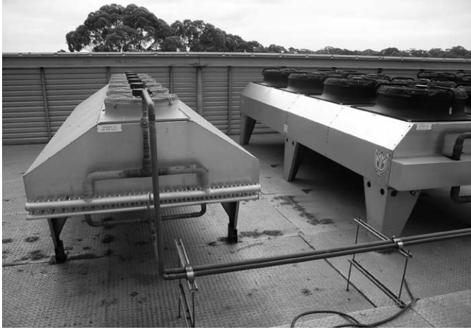
Figure 6.3 A bank of air-cooled condensers
