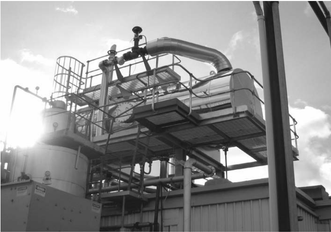
Figure 7.3 A deaerator in an industrial plant
