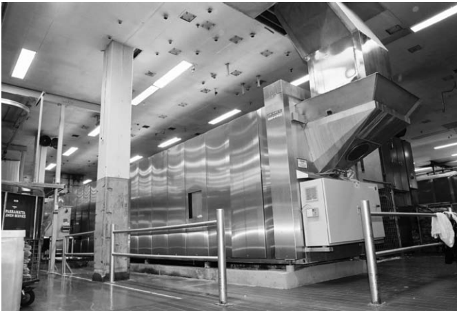
Figure 15.1 A photo of a typical CBW System
