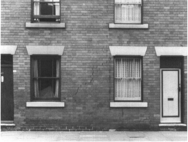
Photograph 3.1: Example of external structural damage caused by mining subsidence (source: British Coal)
