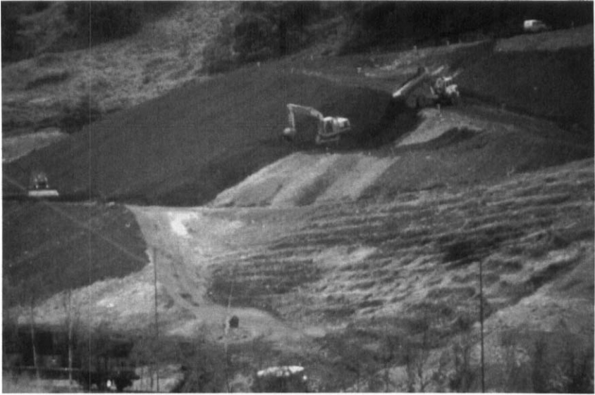
Photograph 14.6: Placing colliery spoil over slag as a growing medium for trees and grass (source: Welsh Development Agency)
