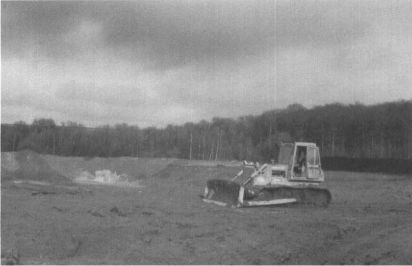
Photograph 17.4: Falquemont. Upper lagoon being filled with ash from the power station (source: Richards, Moorehead and Laing Ltd)
