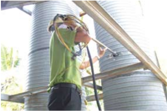
Measuring quality of air emissions from exhaust stack (Source: Thantawan Industry Plc)
