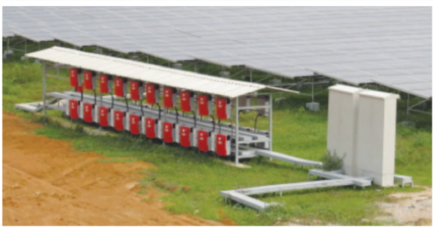
Figure 1: Solar panel used to harness sustainable green energy at Integrated Renewable Energy Park, Pajam, Negeri Sembilan.
