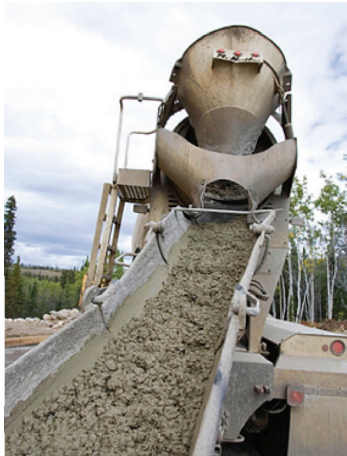
Green concrete, (Image courtesy of Nick Norman / National Geographic RF / Getty Images, Silver Spring Networks)
