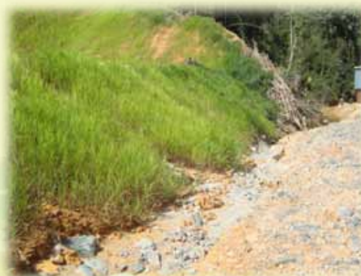
Kawalan perlindungan cerun- "hydroseeding"
