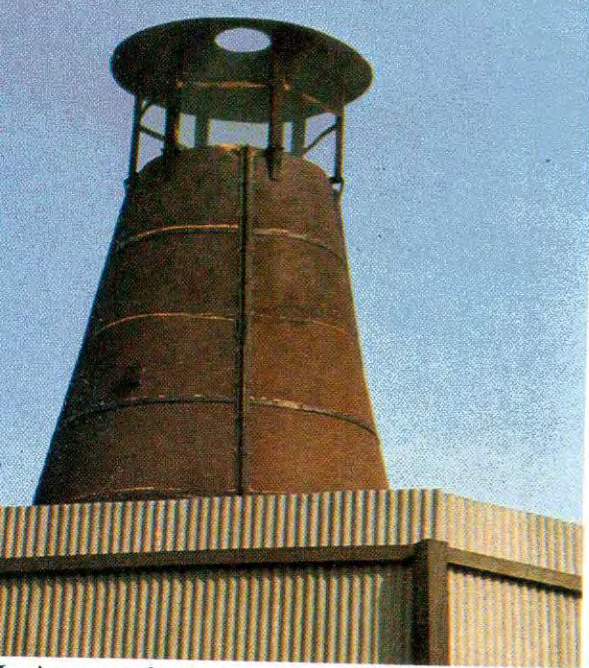
Incinerator for better waste disposal
