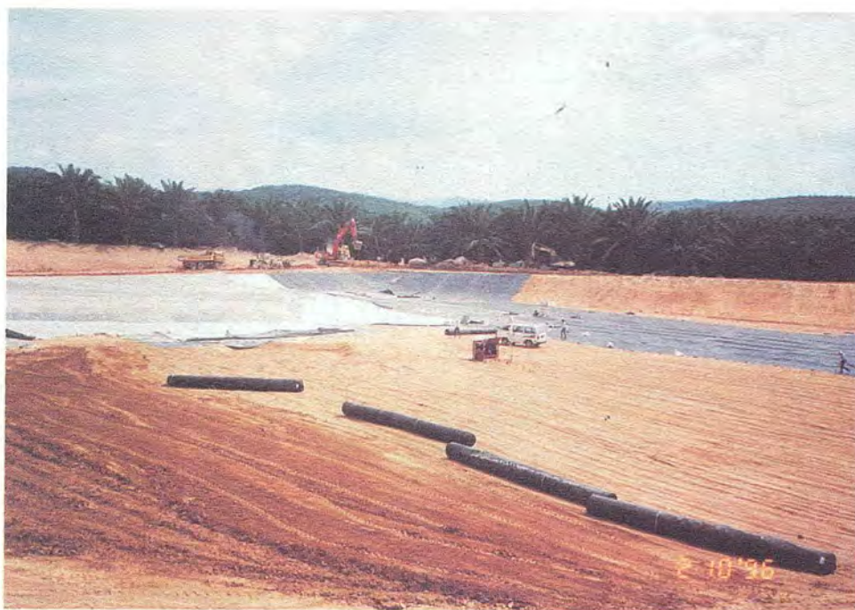
Construction of Secured Landfill Cell at Bukit Nanas, Negri Sembilan in progress.
