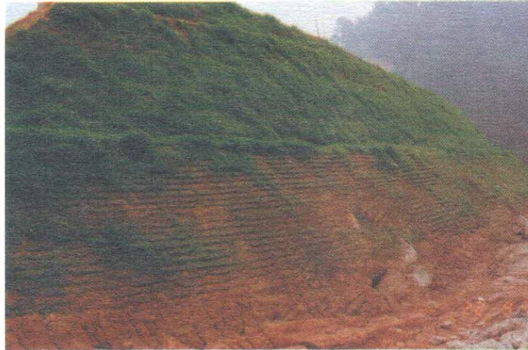
Turfing as a mitigation measure during construction of road at Pos Selim, Perak.
