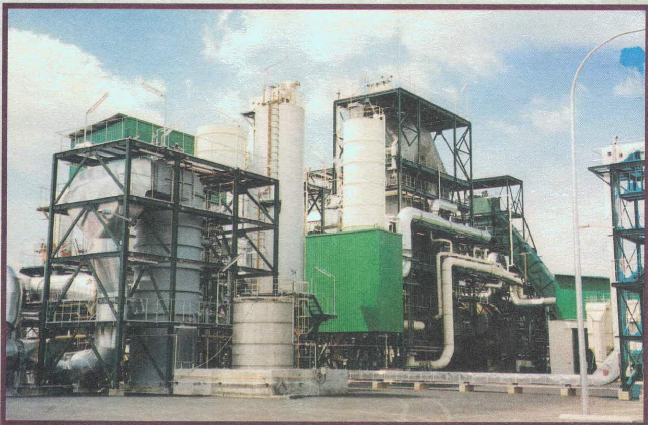
Photo 16: Integrated Scheduled Wastes Treatment and Disposal Facility, Bukit Nanas, Negeri Sembilan (Kualiti Alam Sdn. Bhd.)
