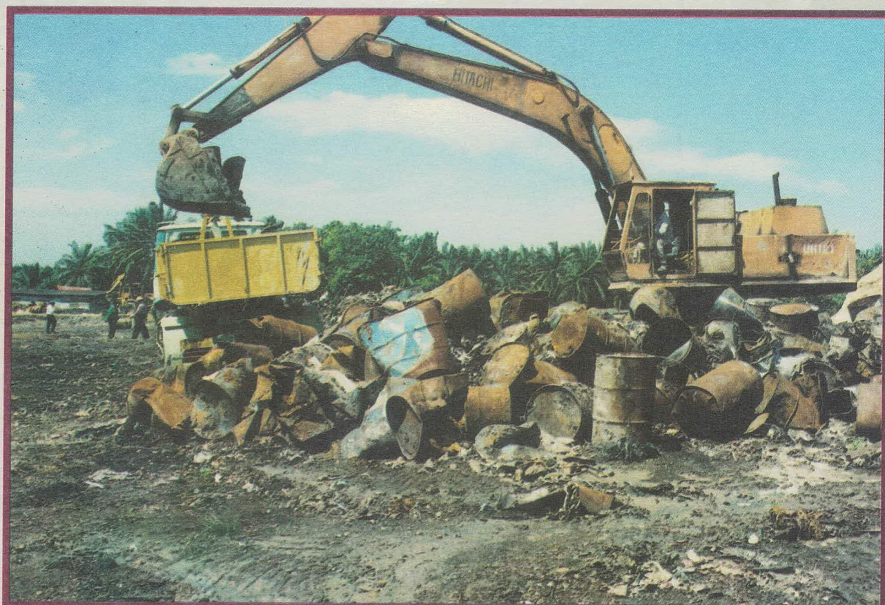
Photo 18: Clean-up of Scheduled Wastes Dumping Site
