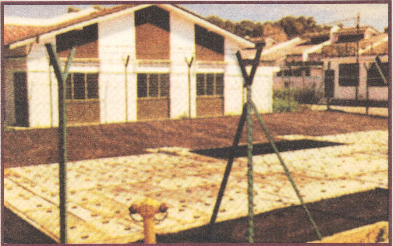
Photo 15: Communal Sewage Septic Tank
