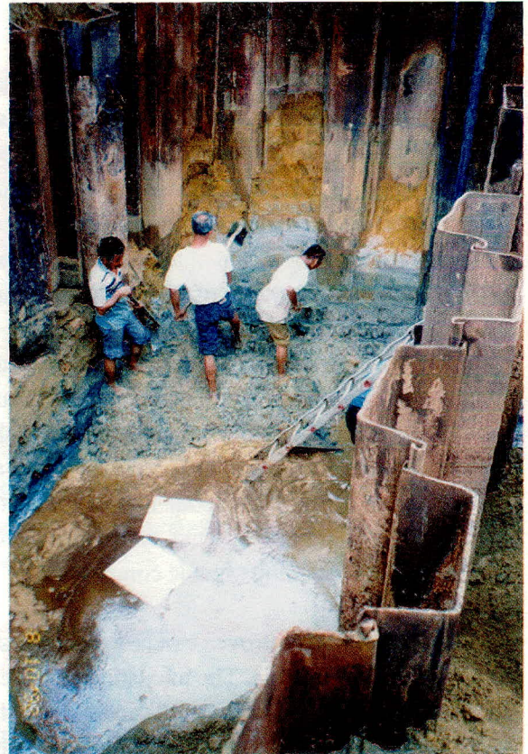
Clean up operation after leak UST have been detected. Leak UST will be taken out and also the contaminated soil and ground water before remedies action are being taken.
