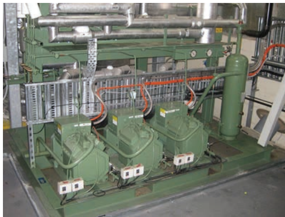
Figure 2.5: Example of Carbon Dioxide (CO 2 ) plant
