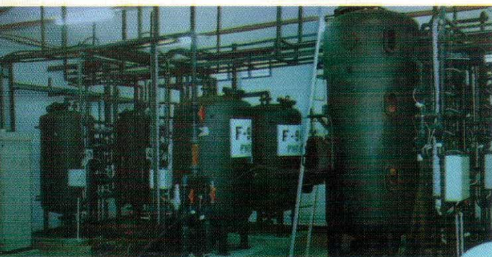
Pure Water Treatment System
