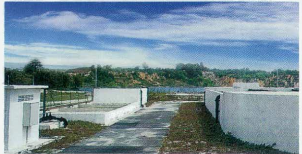
Oxidation Ditch sewage treatment plant for Taman Sungai Besi Indah, Kuala Lumpur, Malaysia.
