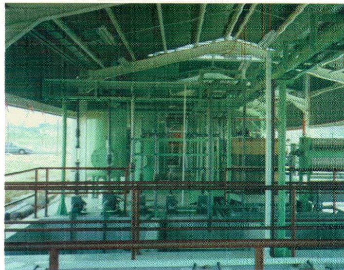
Industrial Waste Water Treatment System
