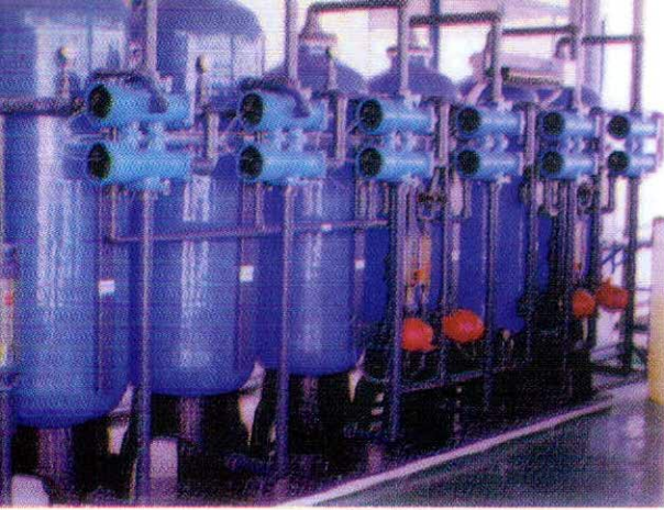
Waste Water Recycle System
