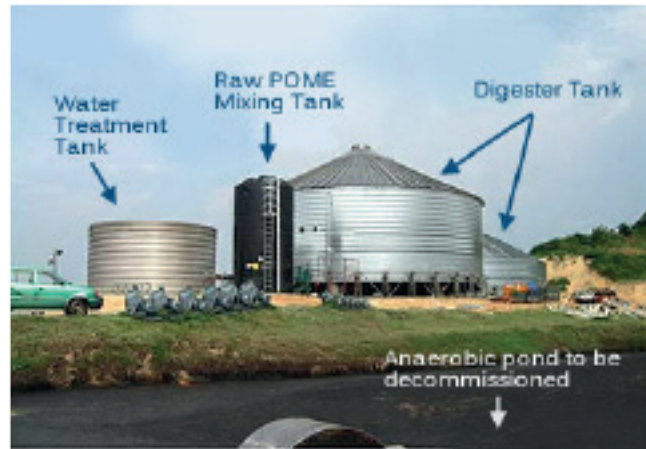
Figure 3.1: Biogas Plant (Example of methane capture from POME)
