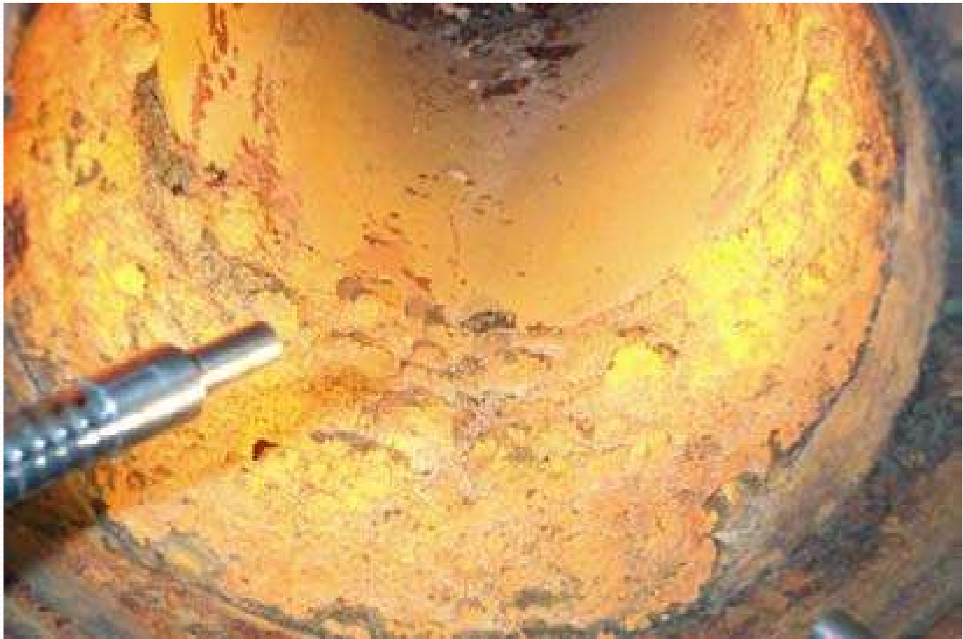
Scale build-up on internal pipe surface
