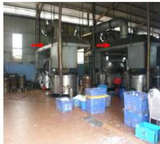
Cooking Area Arrows show the smoke hood
