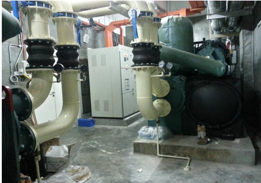
Chiller: 320RT x 2 unit
