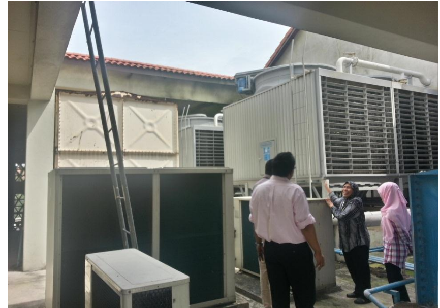
Cooling Tower: 2 unit
