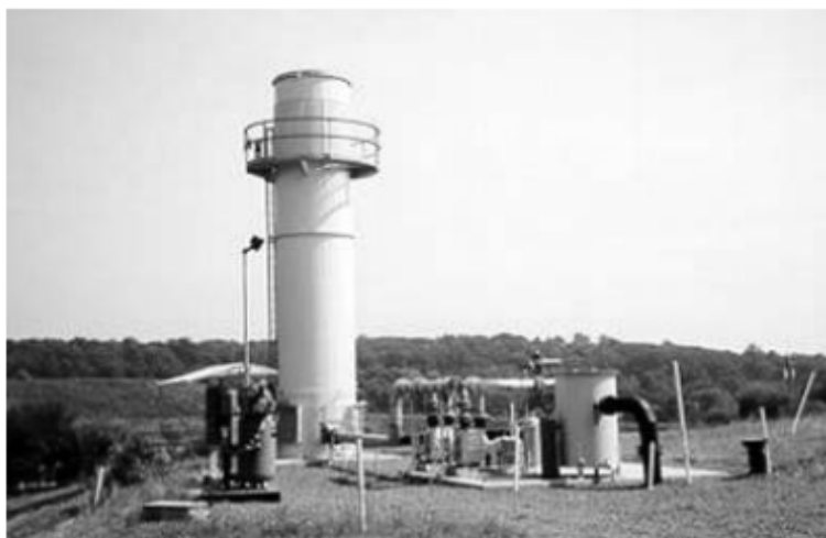
Figure A.11. Typical enclosed ground flare
