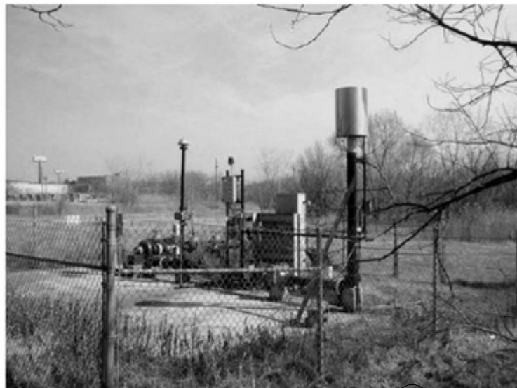
Figure A.10. Typical blower facility.
