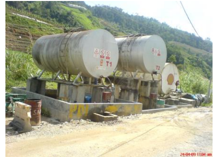
Secondary container with oil interceptor
