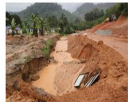
OBSERVE HEAD CUT AND SCOURING
