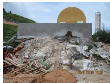
Secondary containment system – wrong application
