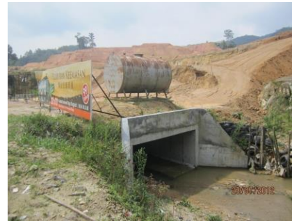
Skid tank: Wrong location and no secondary containment
