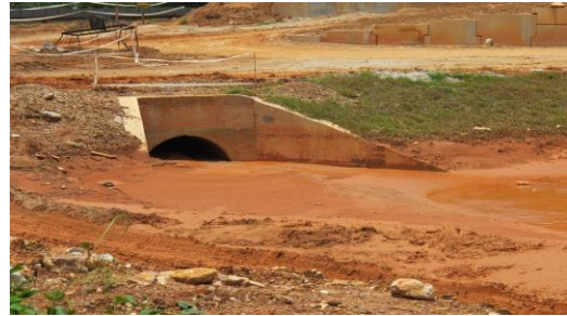
v. Inadequate maintenance provided
