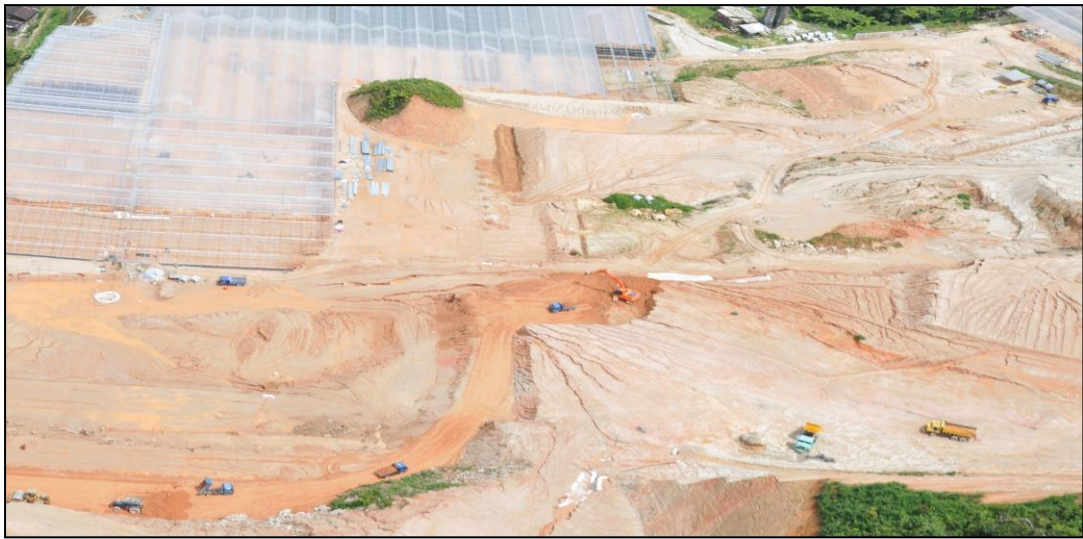
Figure 4.1: Large Scale Earthworks with No Proper BMPs Installed
