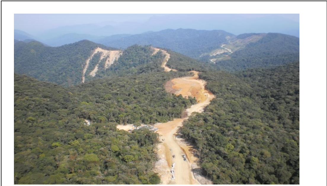
Figure 4.8: No Indication of Works Phasing Implemented
