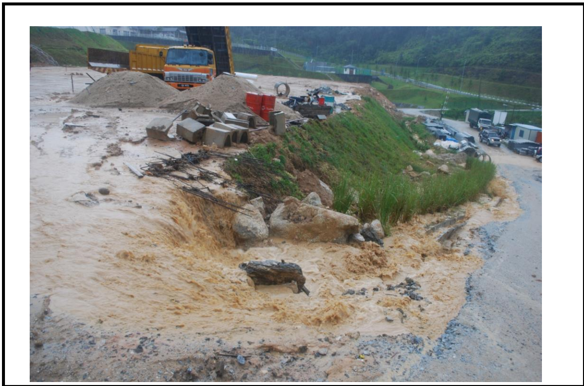
Figure 4.7: Erosion and Surface Runoff from a Poorly Managed Work Site
