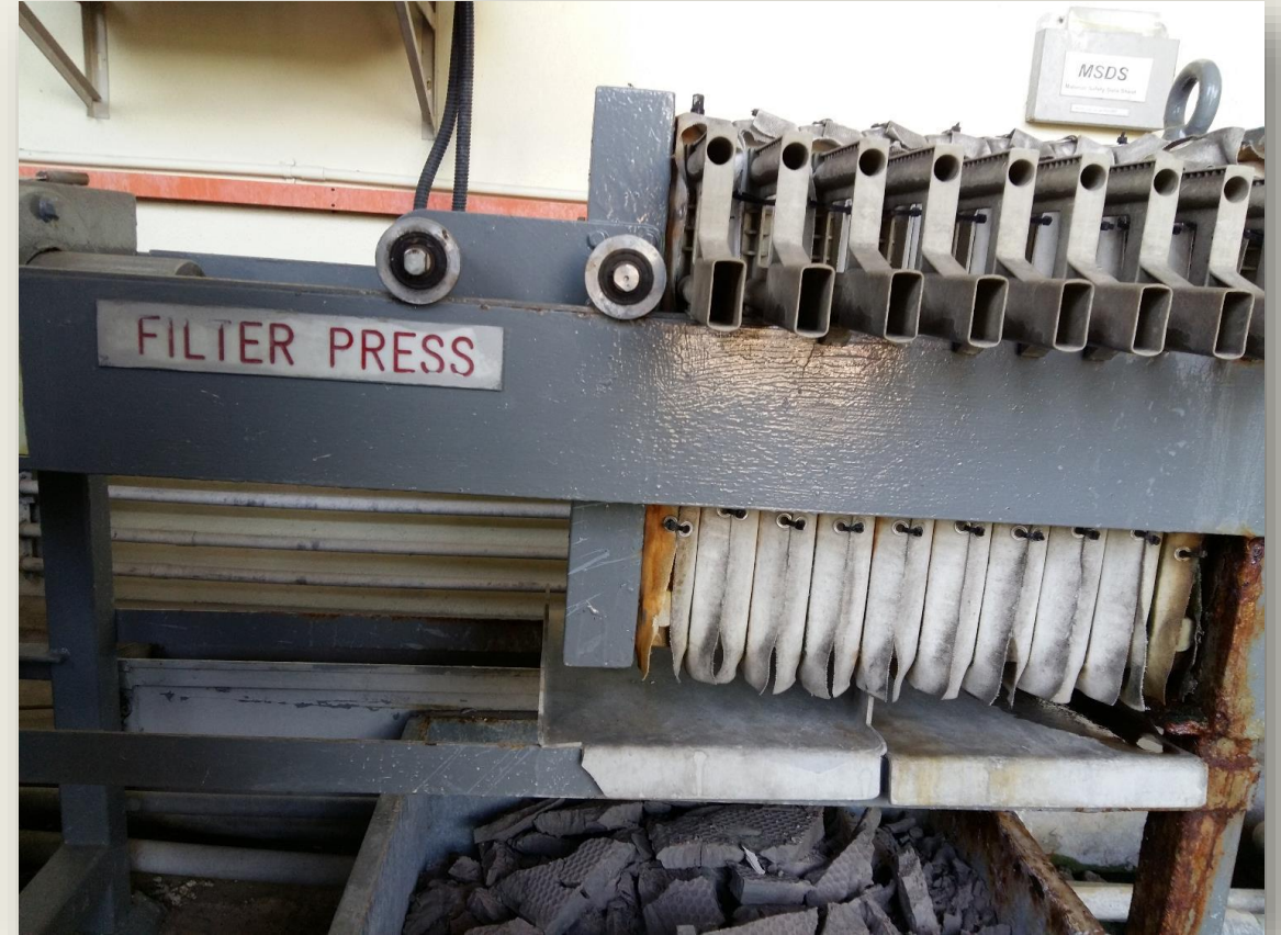
The sludge the is being filtered in the filter press.
