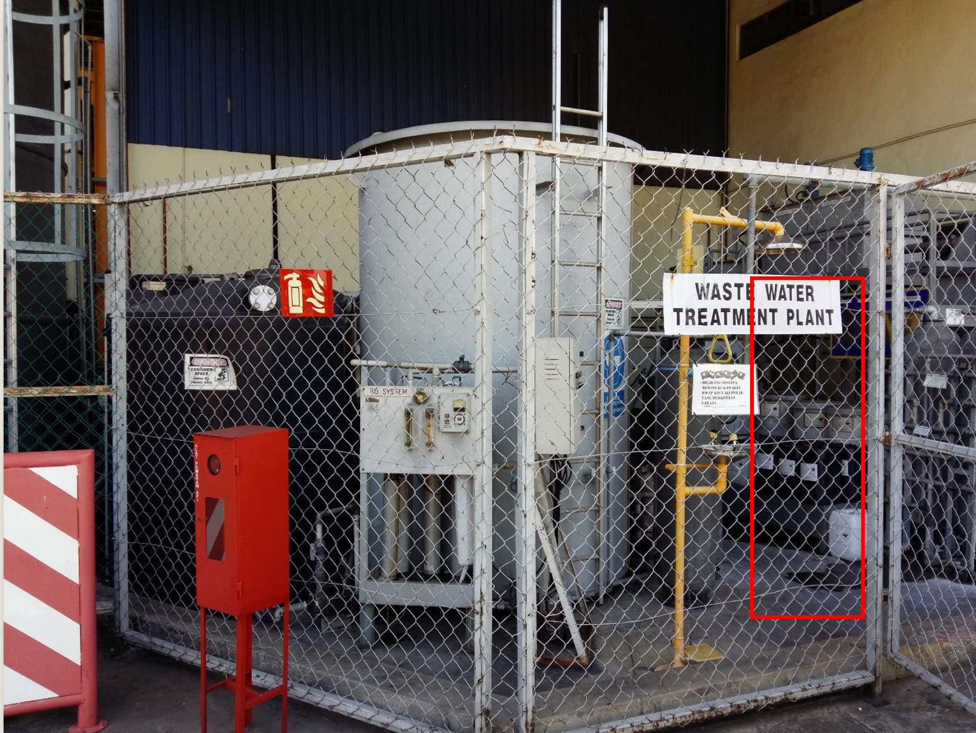
The activated carbon filter of WWTP at EMERSON.
