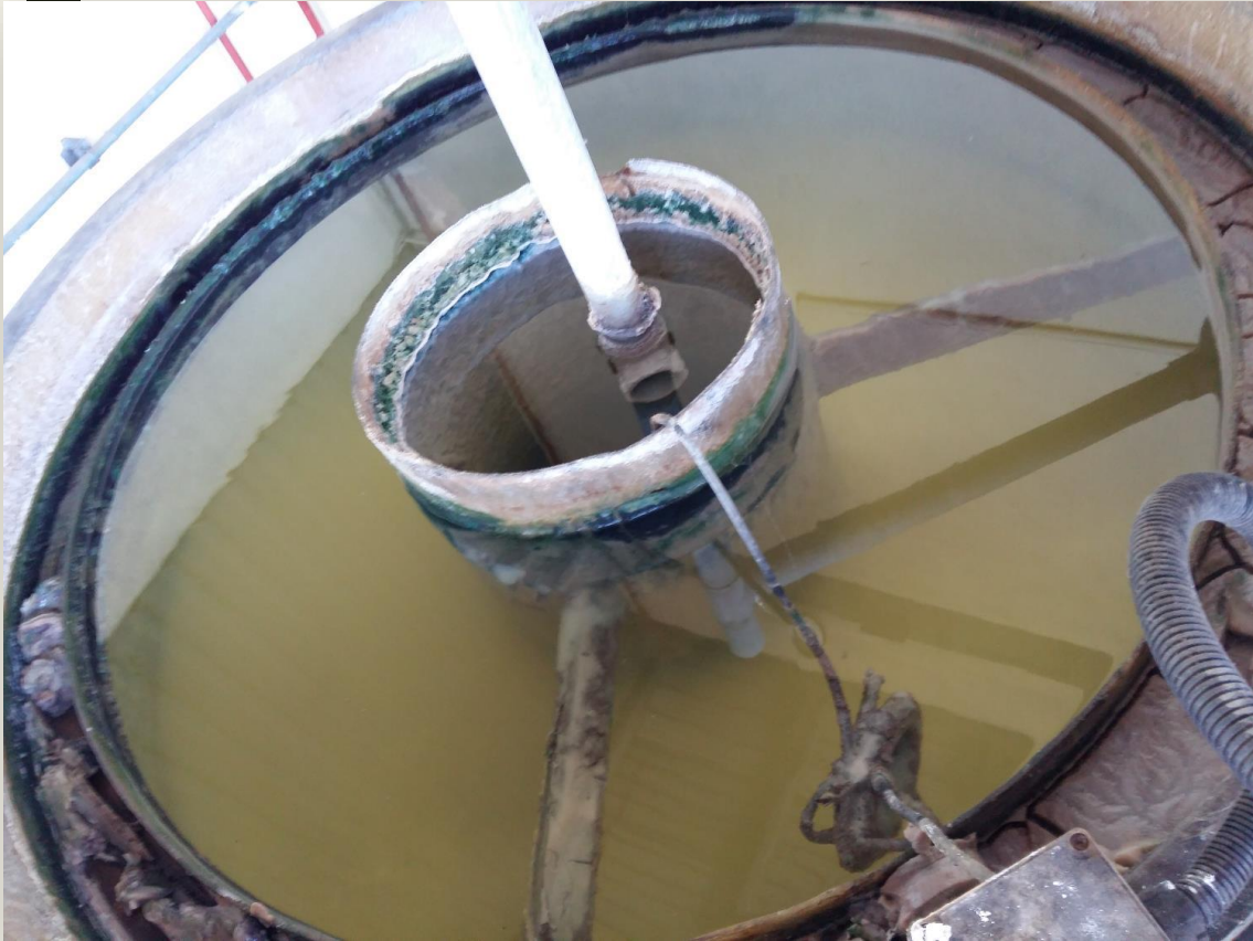
Sludge thickening in the sludge thickener tank.
