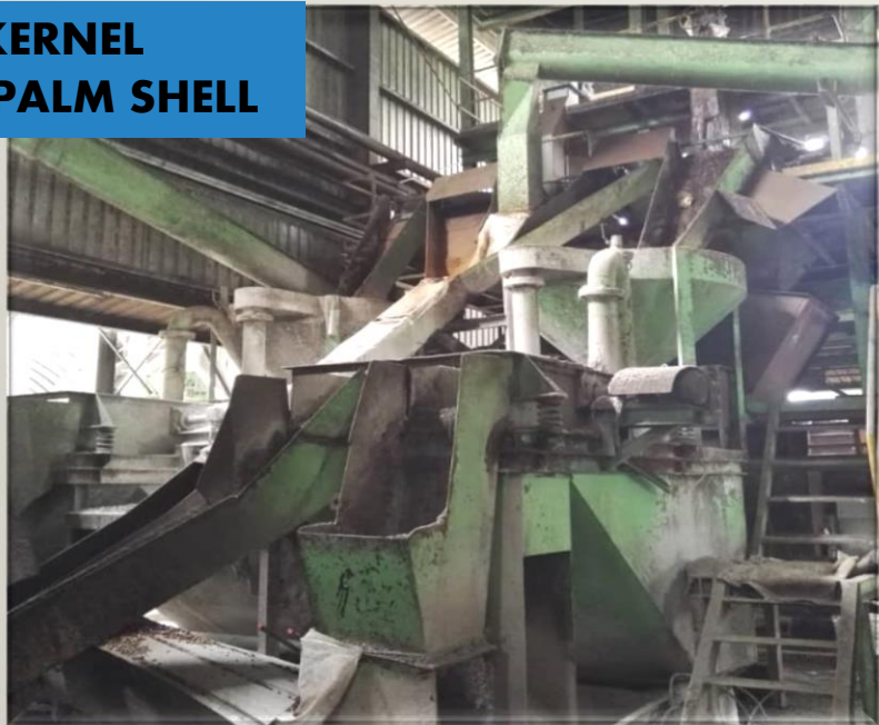
HYDRO CYCLONE & CLAYBATH
