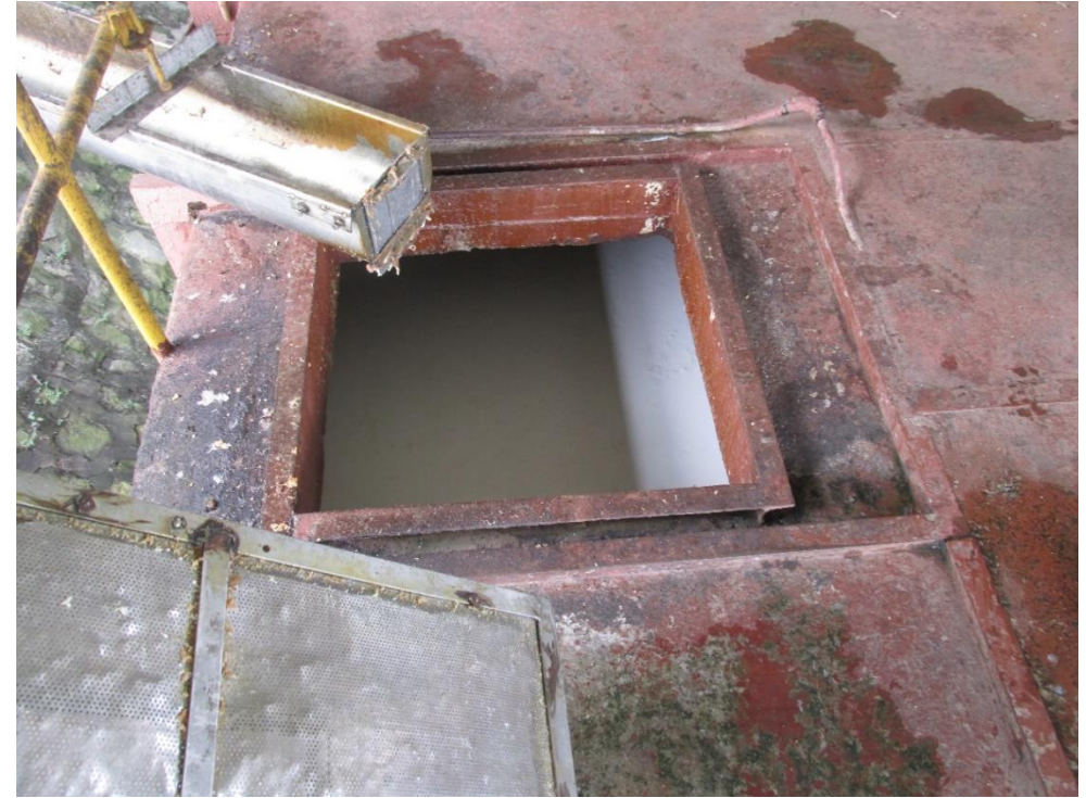
BULKING TANK – PROSES PENCAAMPURAN PREVULCANIZED & FRESH LATEX
