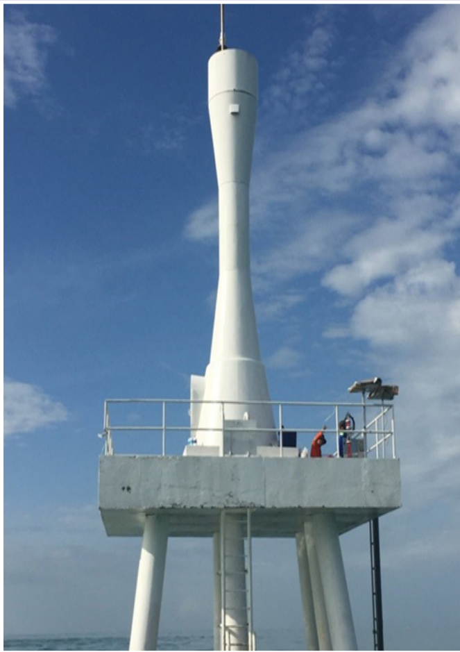
▶ Stesen Pengawasan Kualiti Air Marin Automatik The Continuous Marine Water Quality Monitoring station
