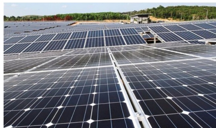
Solar PV for electricity generation
