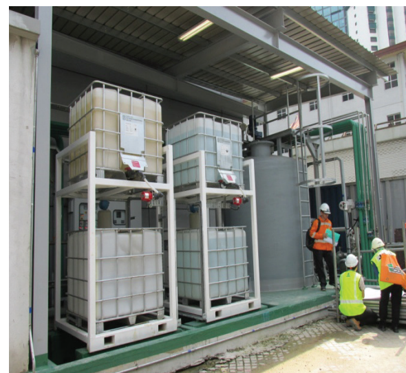
Gambar 3(i) : Loji Rawatan Efluen Perindustrian bagi Cooling System
