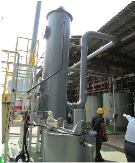
Gambar 3(j) : Alat Kawalan Pencemaran Udara Scrubber
