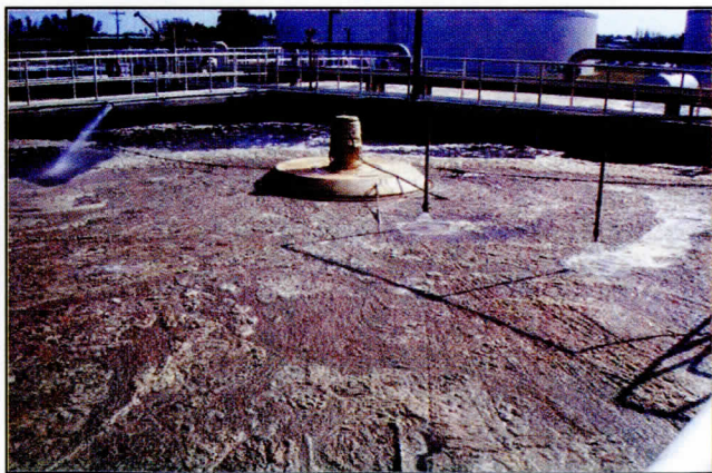
Figure 4.2 Sludge bulking in an activated sludge process (Source : http://www.qmes.nl )
