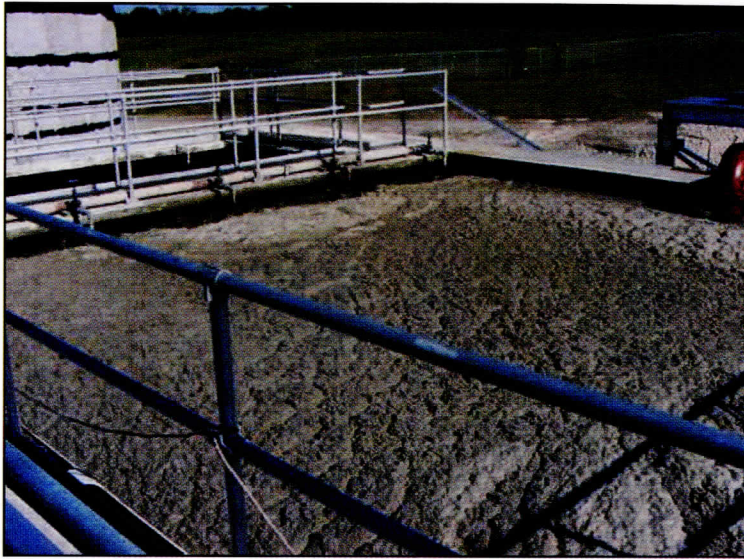
Figure 4.9 Foaming in the aeration tank (Source : http://www.tpomag.com )
