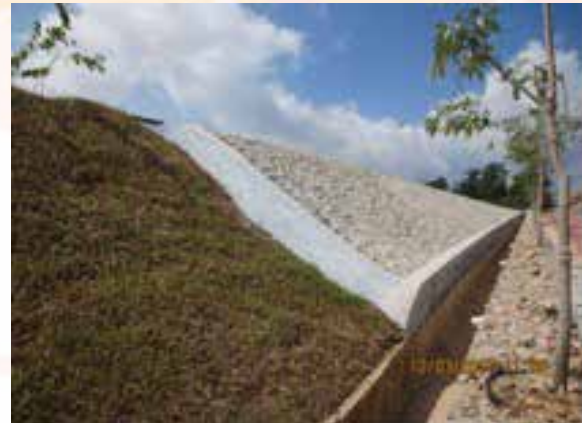
Kawalan perlindungan cerun ( Stone pitching dan close turfing )
