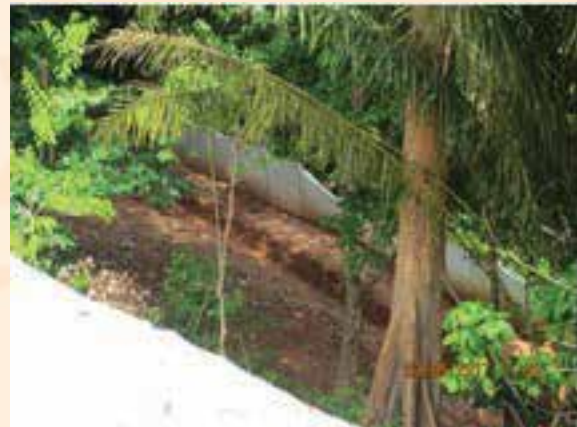
Kawalan Pencemaran Air Larian Permukaan ( Silt fence )
