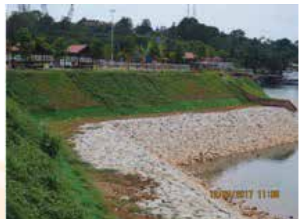
Kawalan Perlindungan Cerun ( Rock revetment )
