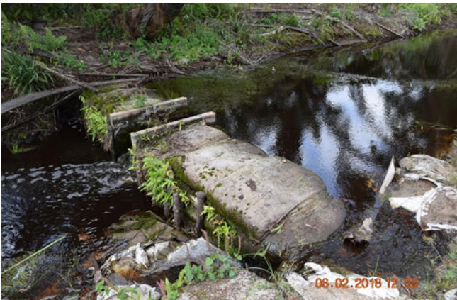
Gambar 4.24 JAS Negeri Johor: Check Dam Geobag
