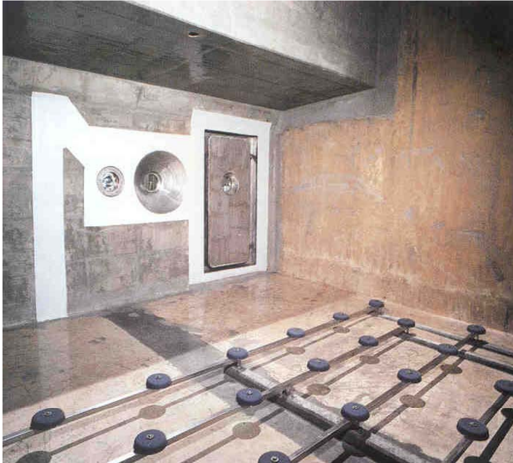
Figure 3: View inside a diffusion chamber, the ozone gas enters the chamber through diffusers
