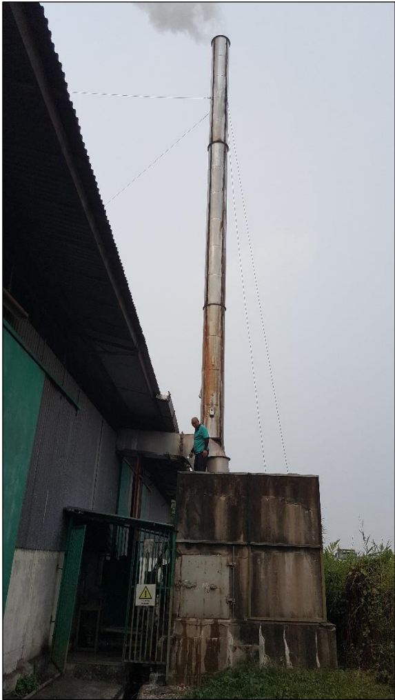
(c) The wet scrubber at a feedmill had a poor odour removal efficiency of 26%, which still emitted 3048 OU/m 3 after undergoing treatment. This scrubber was feed with water extracted from the nearby river as part of the system operation.
