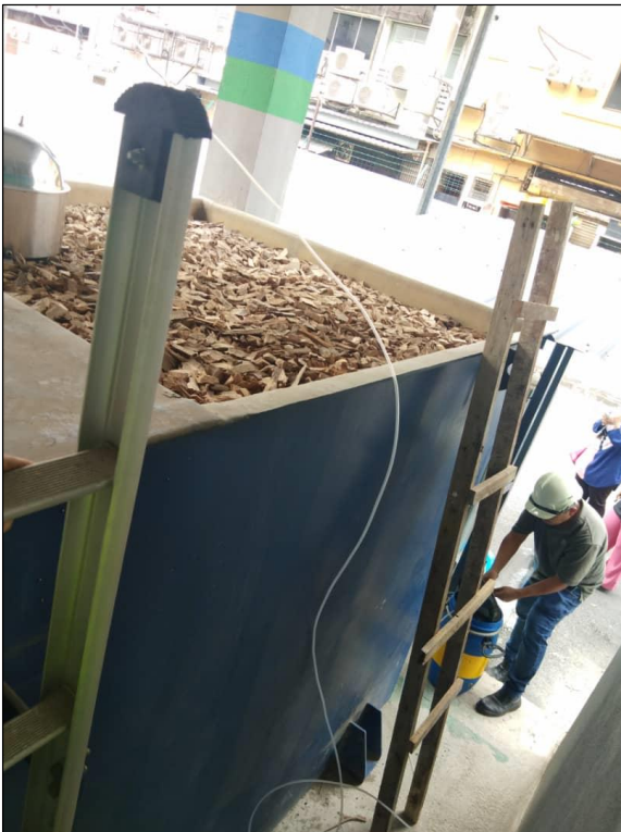
Figure 5.2 (a) The biofilter at a sewerage pump station was emitting an average 158 OU/m 3 from its treatment system.
