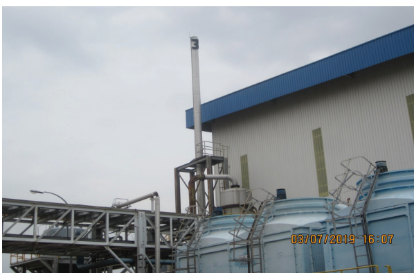
Alat Kawalan Pencemaran - Cerobong
