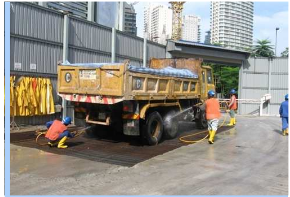
Wheel Washing Facilities
