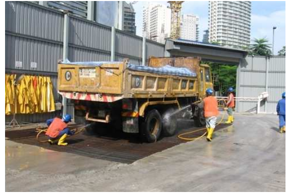
Wheel Washing Facilities
