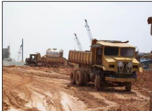
Poor worksite management
