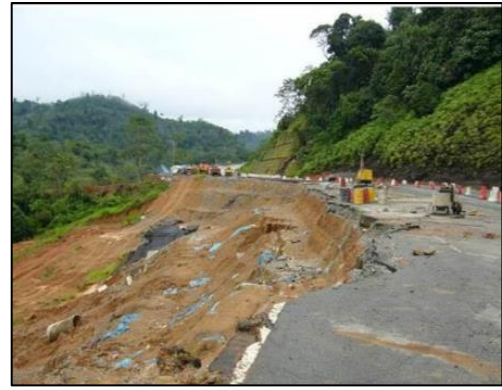
Landslides and mudflows
