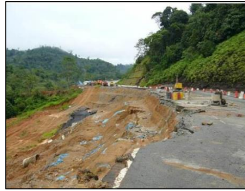
Landslides and mudflows
