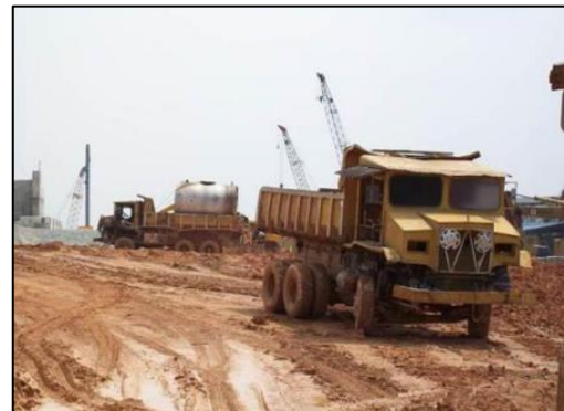
Poor worksite management
