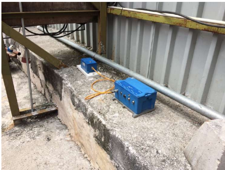
Plate B-12: Vibration monitoring unit and accelerometer sensors bolted onto ground beam at perimeter boundary of construction work site
