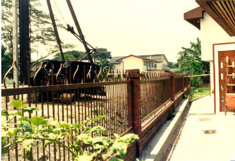
Plate D-1: Drop hammer impact piling works at condominium project site next to existing residential houses
