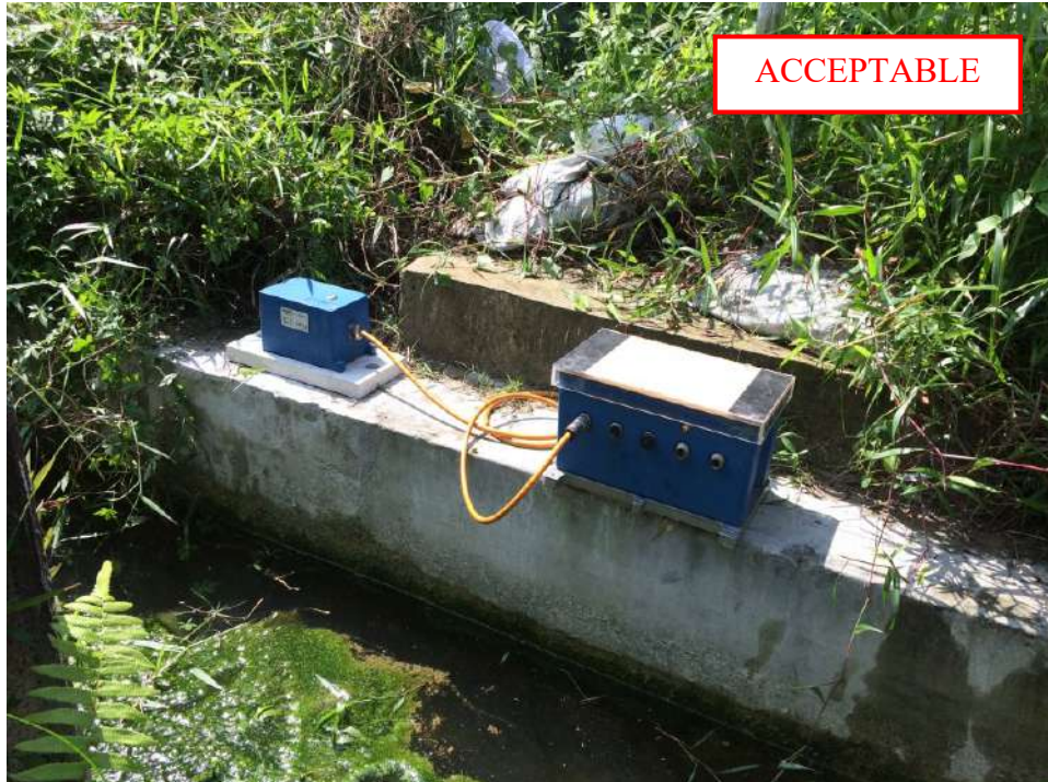
Plate B-25: Vibration monitoring equipment secured onto solid ground beam at residential locations
