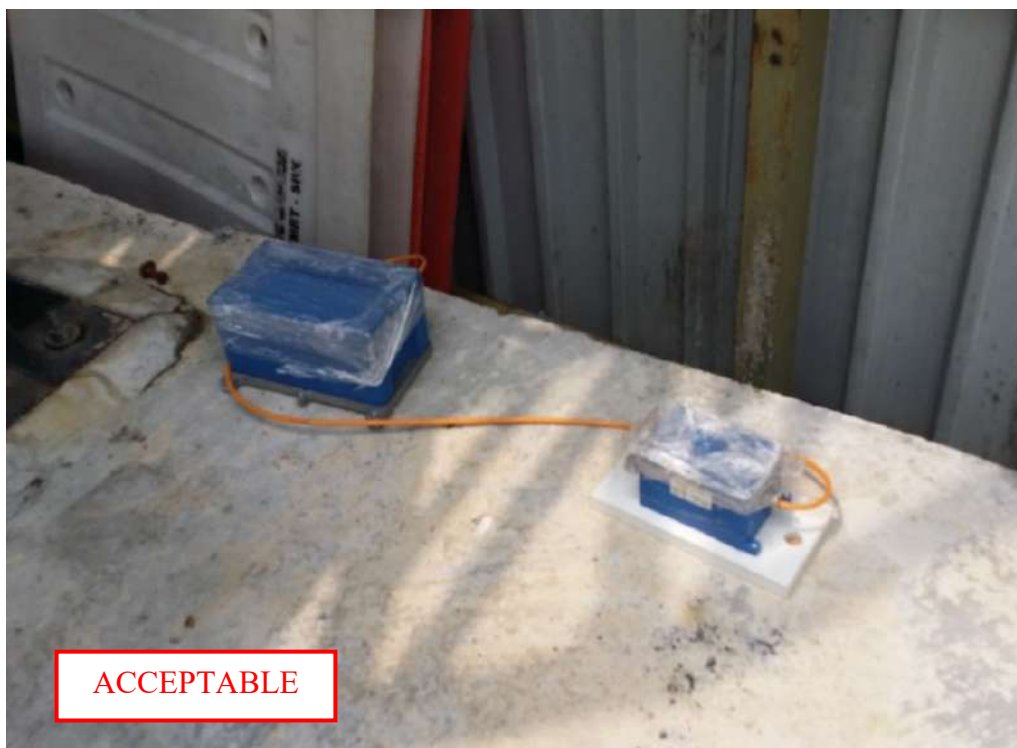
Plate B-18: Accelerometer sensor secured onto mounting plate bolted onto concrete slab
