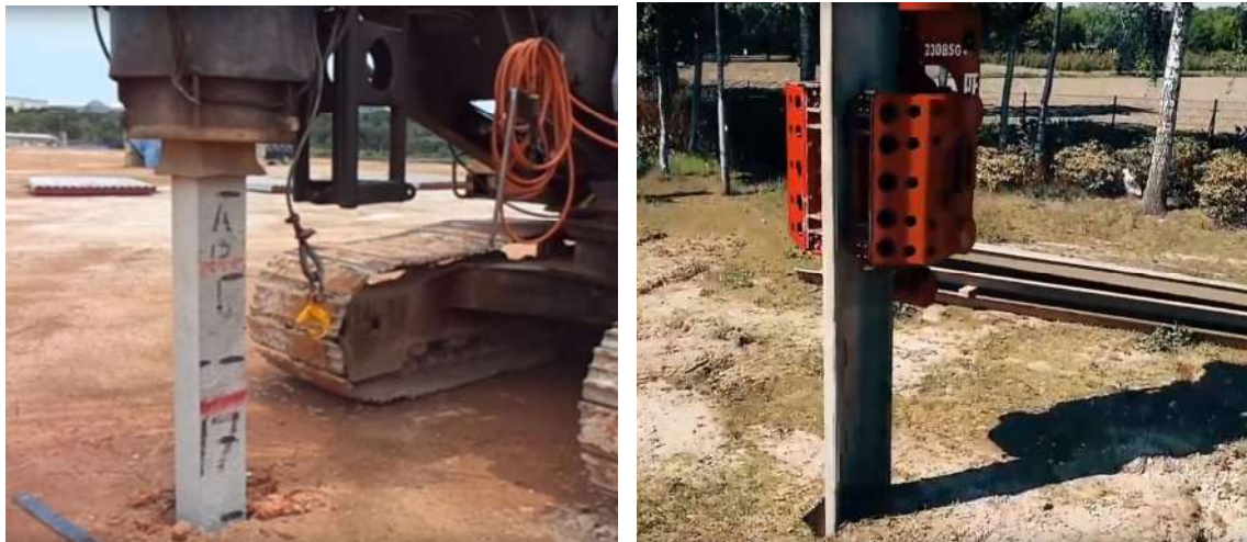
Plate E-3: Examples of (a) typical drop hammer impact pile driving of precast concrete pile; and (b) vibratory hydraulic piling of sheet pile
