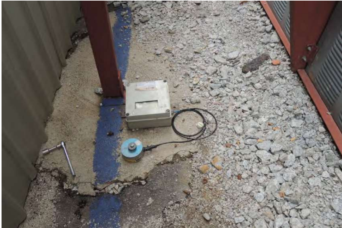
Plate B-13: Vibration monitoring unit and geophone sensor being set up for measurement at construction work site. Geophone sensor rigidly secured onto solid surface with bolt threaded thru sensor body.
