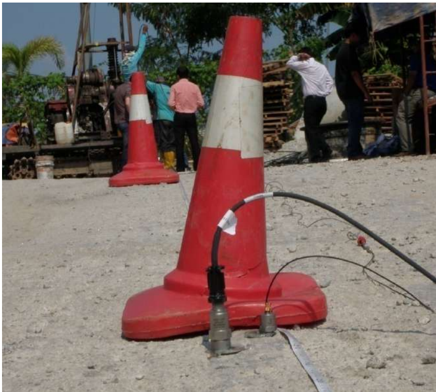
Plate B-14: Vibration sensor (piezoelectric type) with magnetic base secured onto steel washers bonded onto hard ground with epoxy for vibration transfer function testing
