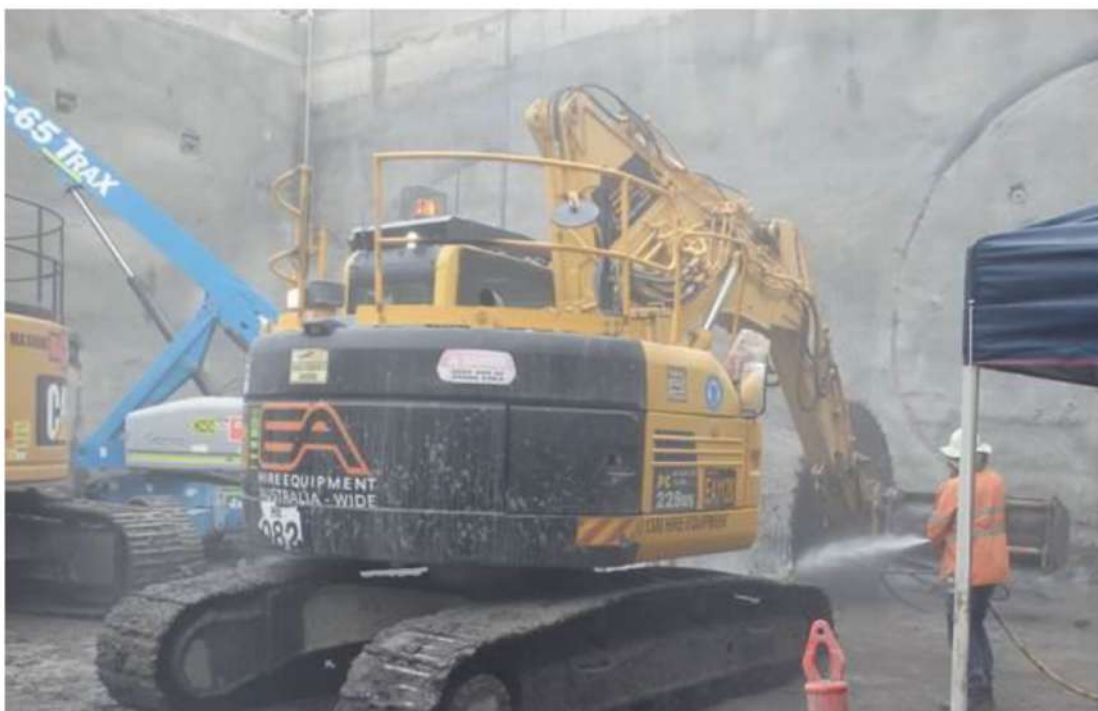
Plate E-20: Rock cutting work in progress in an underground metro project (Australia)
