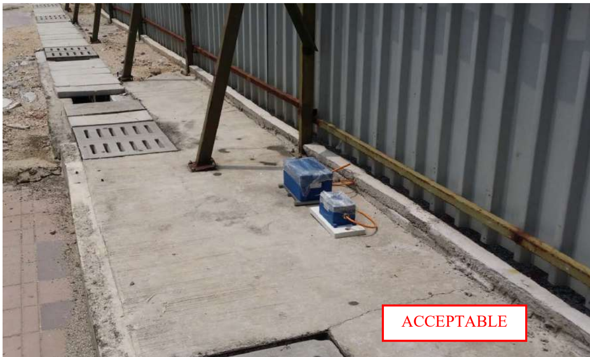
Plate B-20: Vibration monitoring undertaken at construction site perimeter boundary with sensor rigidly coupled onto concrete pavement
