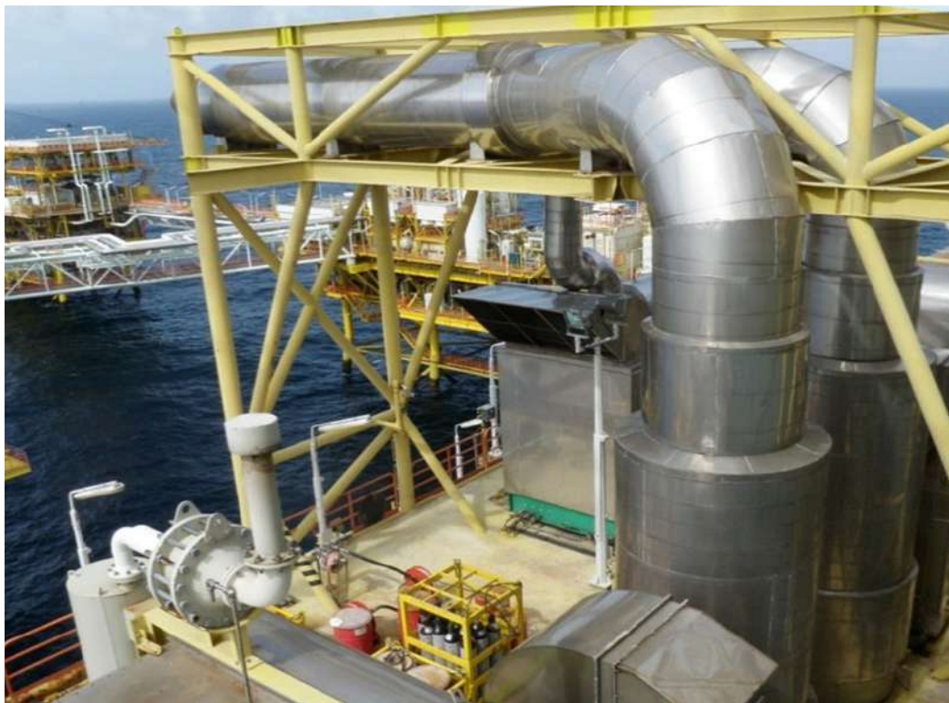
Figure E-21: Reactive silencers used in exhaust noise mitigation
