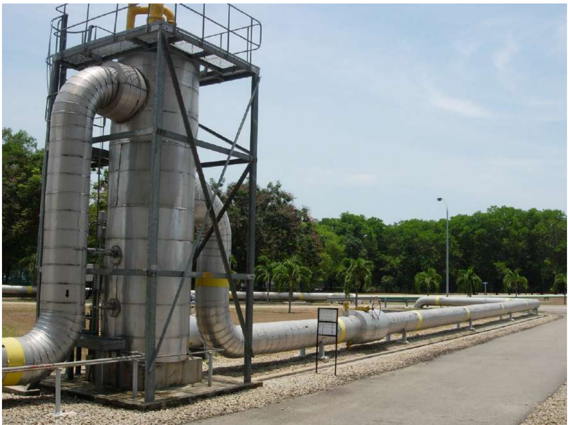
Figure E-26: Example of gas pipes external lagging in industrial noise mitigation
