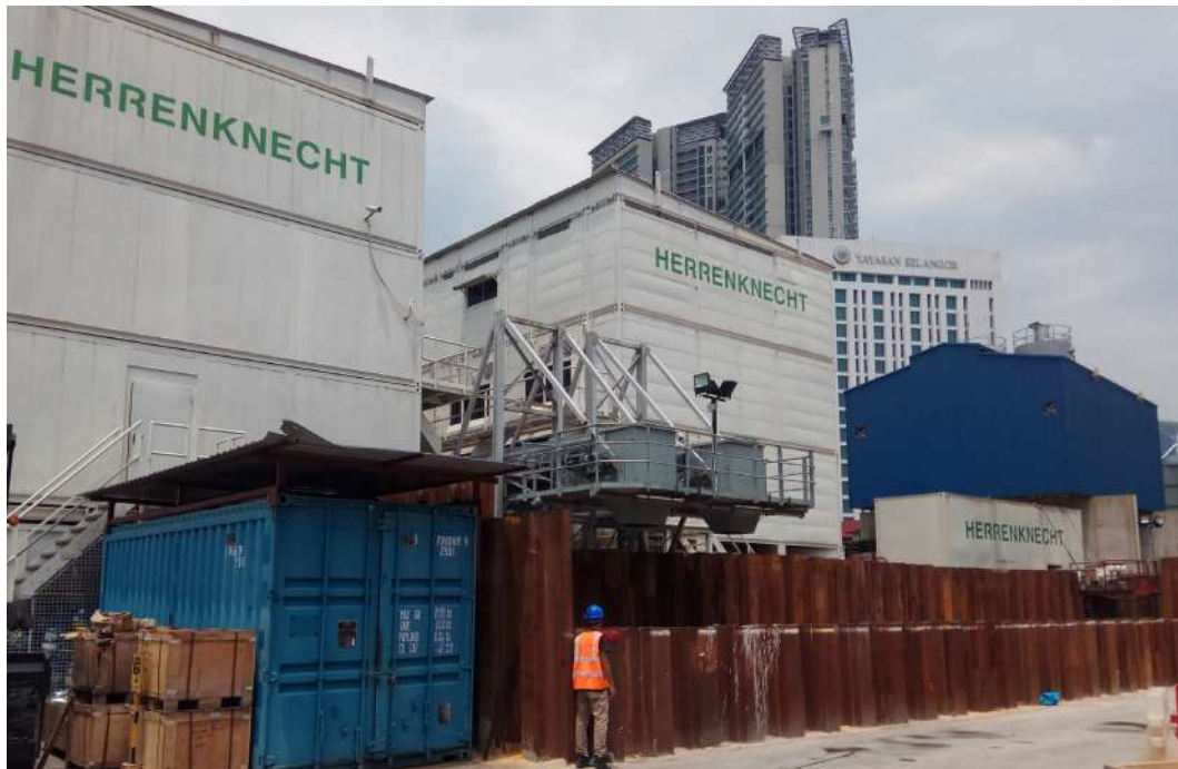
Figure E-15: Full enclosure for slurry treatment plant in Klang Valley MRT construction work site adjacent sensitive receptors
