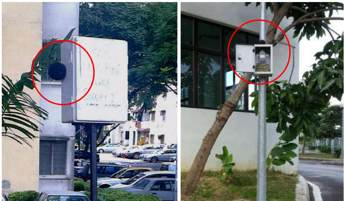
Figure B-15: Examples of unacceptable use of sound level meter installed in a casing as an alternative to permanent noise monitoring units
