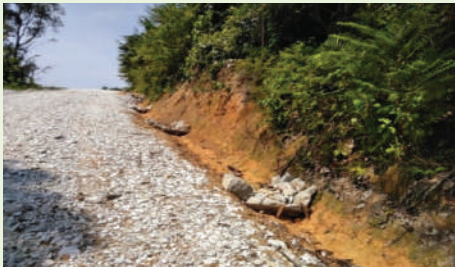
i. Check dam along the earthdrain with wood stack as anchoring mechanism at steep slope area
