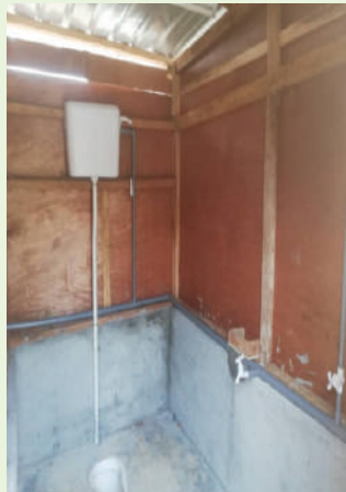
ii. Temporary site cabin toilet
