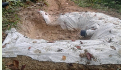
ii. Discharge pipe from silt trap covered with on the inlet point
