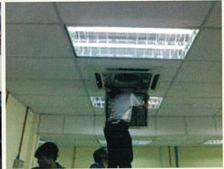
Maintenance is important to ensure the system operate efficiently
