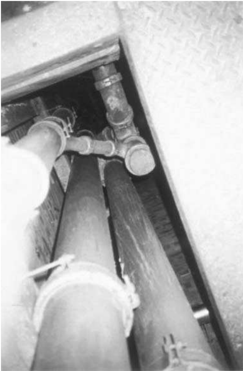
Figure 7.6 Modified one-pipe drainage and vent system in a service shaft at the Queen's Medical Centre, Nottingham (Courtesy of Schott UK Ltd)
