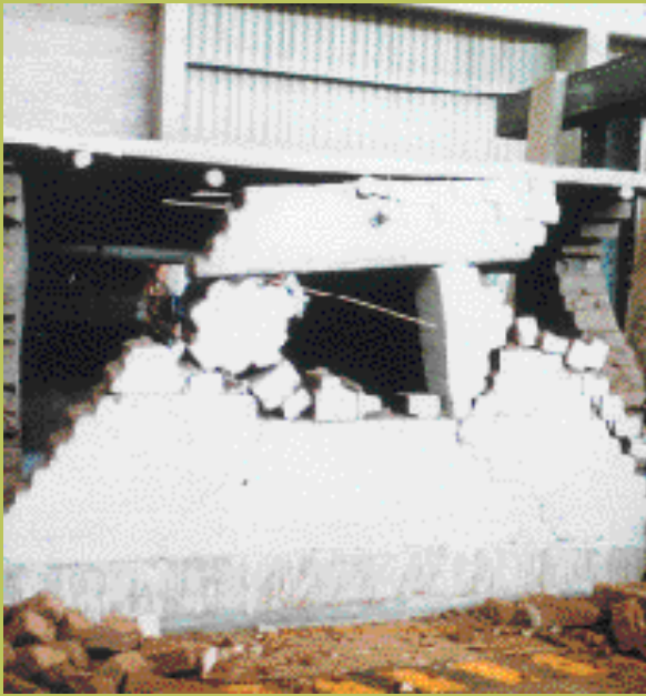
Figure 2: Collapse of unreinforced module...
