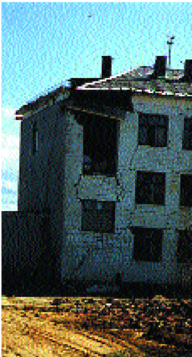
Figure 2: The partially damaged school building in Neftegorsk
