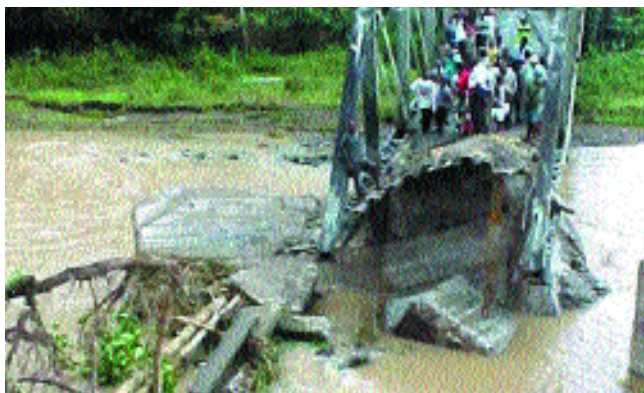
Damage caused by the St Mary's flood rains, 18 May 1999
