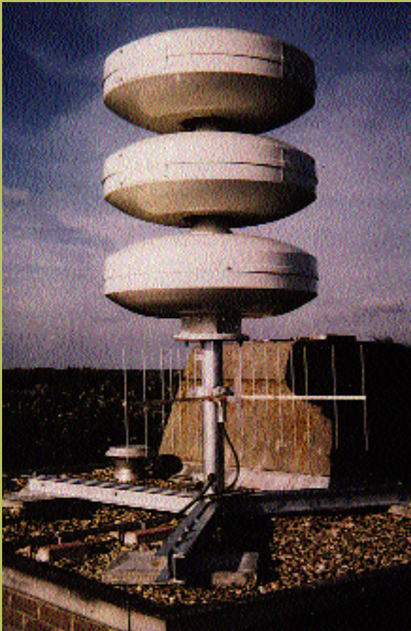
The actual activation of the sirens is achieved by a radio signal through one of the communication networks of the fire service organisation
